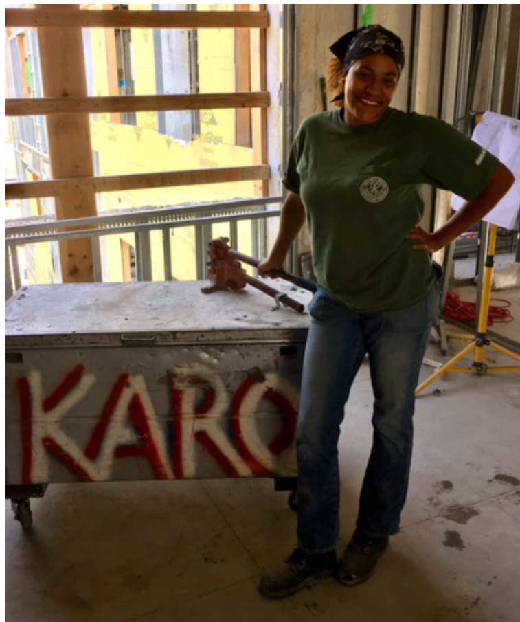
Linette Hooker, second term sheet metal apprentice, Local 28, working at the reconstruction of NoVo Foundation's new NYC HQ
